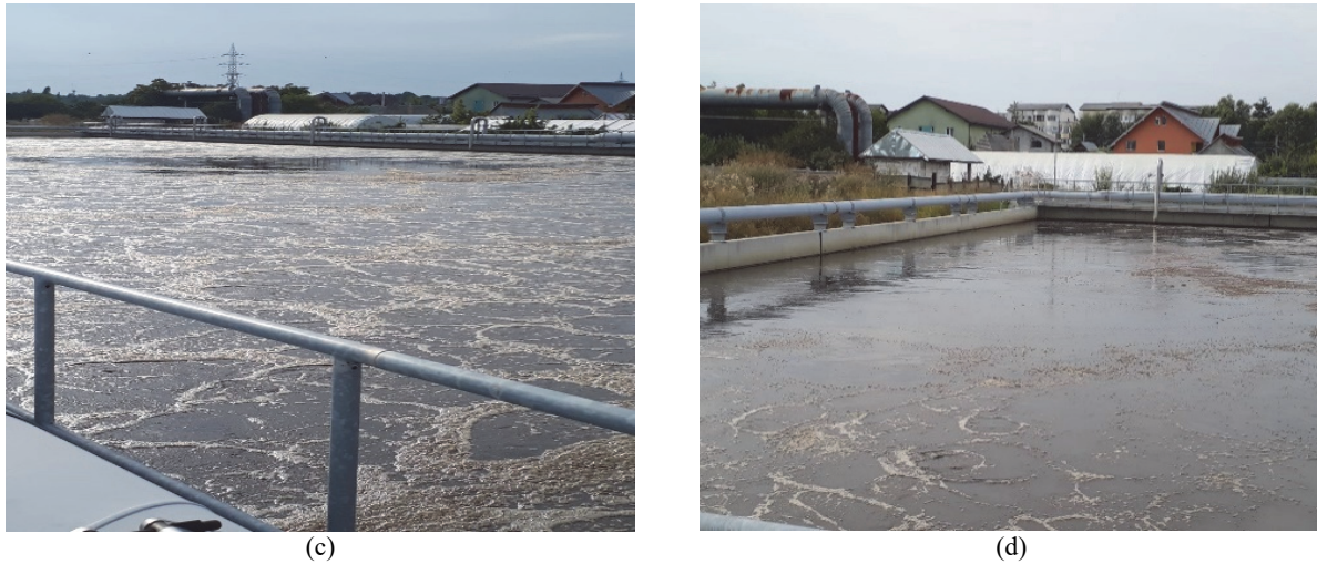
Fig. 6. (a) Dislodged porous diffusers; (b) Flow regime in bioreactor; (c) "Dead water" zones in bioreactor; (d) "Dead water" zones in oxic zone
