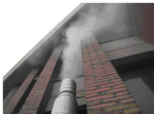
Fig. 4. Monitoring the smoke aspect at the stack
