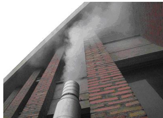
Fig. 4. Monitoring the smoke aspect at the stack
